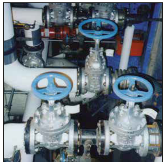
Gate valves in service for a boiler feed installation.
